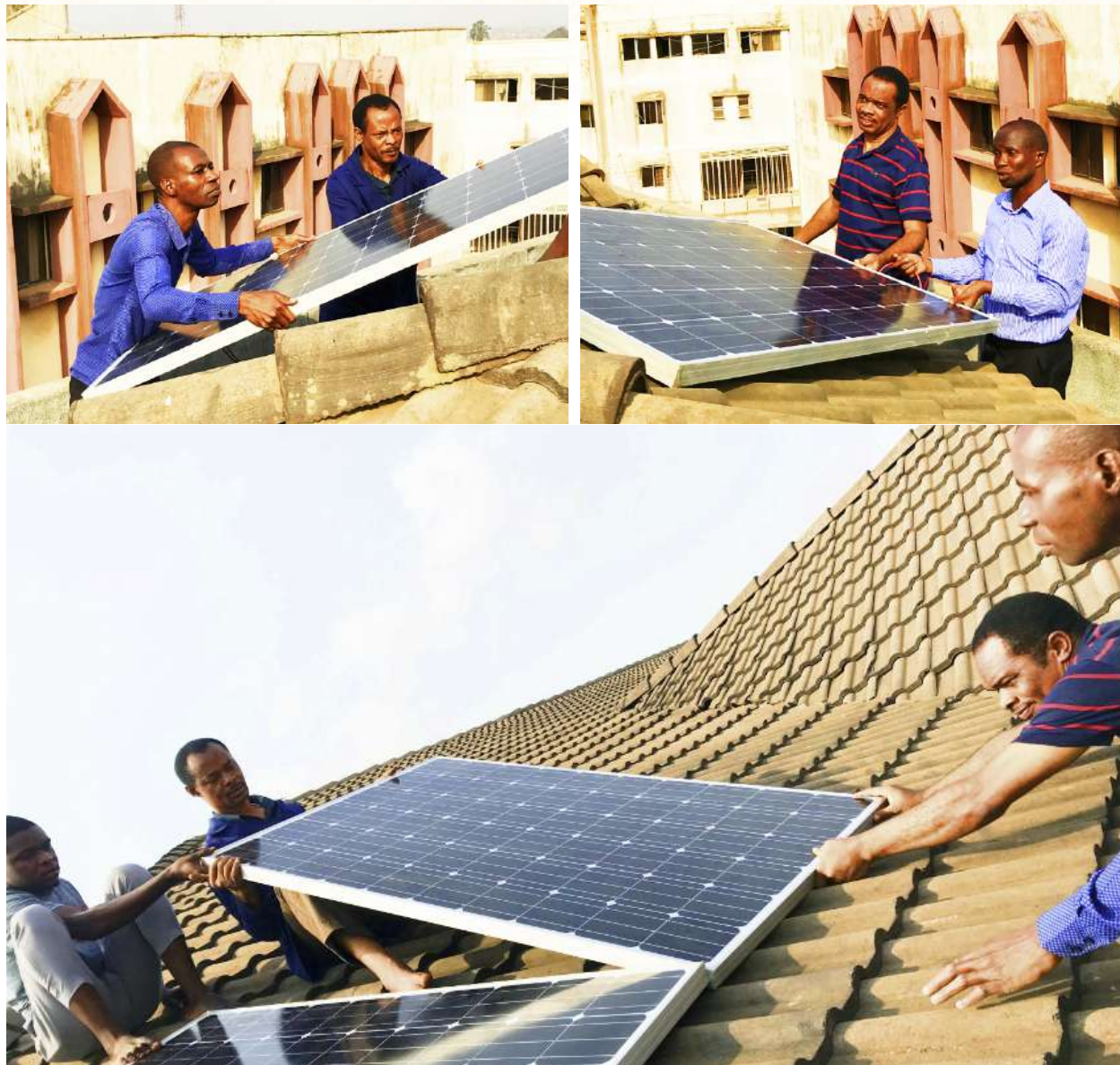
Members of the Space Lab research team installing the solar panel system for the lab.
